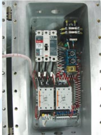
REVERSING STARTER FOR CONVEYOR AUGER RIG MUD SYSTEM
