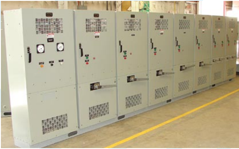
DC SWITCHBOARD 3000 AMP / 125 VDC UPS AND BATTERY DISTRIBUTION PANEL
