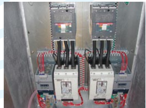
DUAL 100 HP SOFT STARTERS IN NEMA 7 ENCLOSURE
