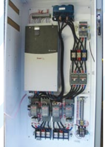
VFD DRIVE UNIT FOR 150 HP STEAM BOILER SYSTEM
